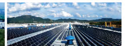
Solar panels arrays
